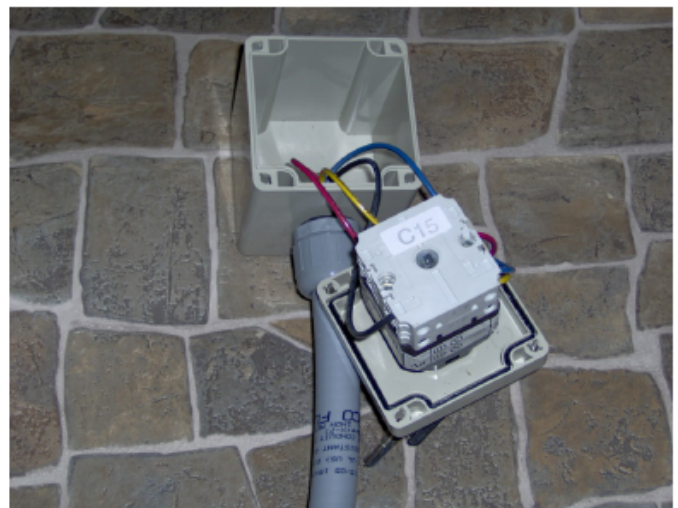
4 x 14 gauge wires used for key switch
